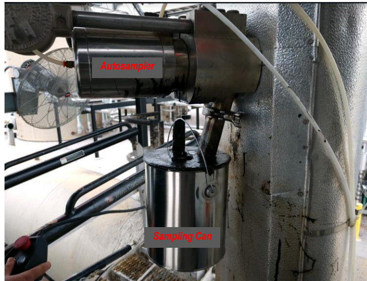
Figure 6 An Autosampler Device Installed towards the End of a Loading Pipeline
